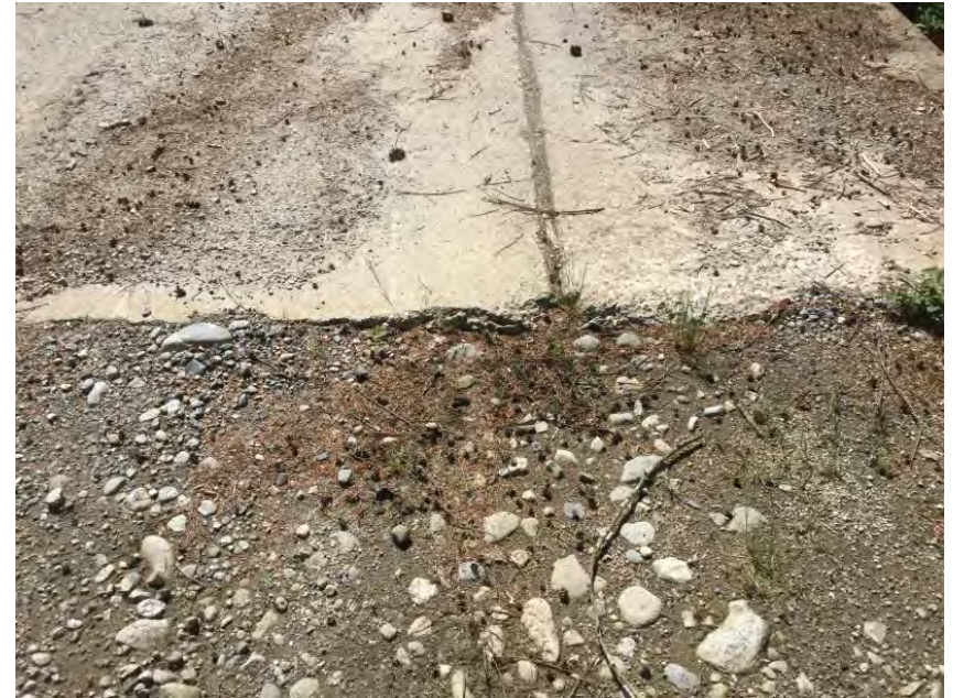
Minor damage noted at right approach
